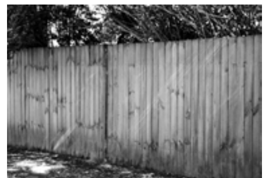
▲ Palings damaged by contact with the ground
