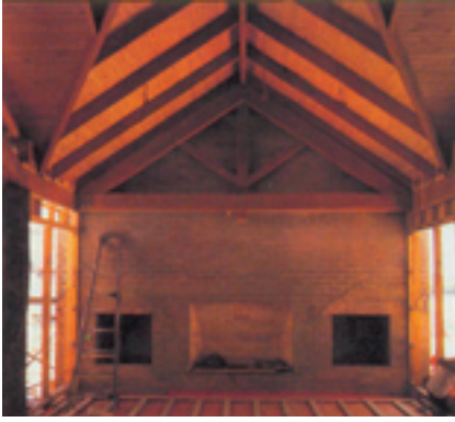
Seasoned 45 mm x 70 mm bearers fixed at 450 mm centres over a cured concrete slab
