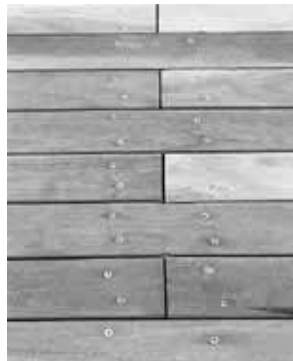
Fig 22 Staggering of plank joints in wide sections of decks is facilitated by paired joists
